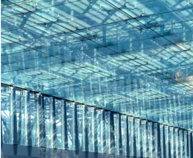
The 113 x 36 m (370,73 x 118,11 ft) roof of the Endesa HQ comprises an almost horizontal flat glass surface composed of 861 point-fixed laminated glass panes, with a total area of approximately 3,150 m 2 (32,000 sq ft).
